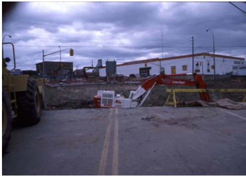
Remedial work project on an abandoned mine beneath a major city intersection
